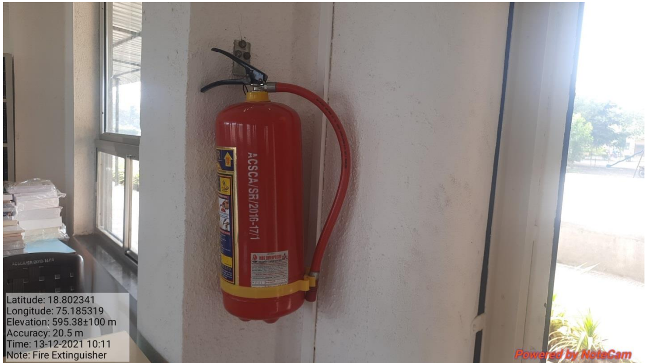
Library Fire Extinguisher
