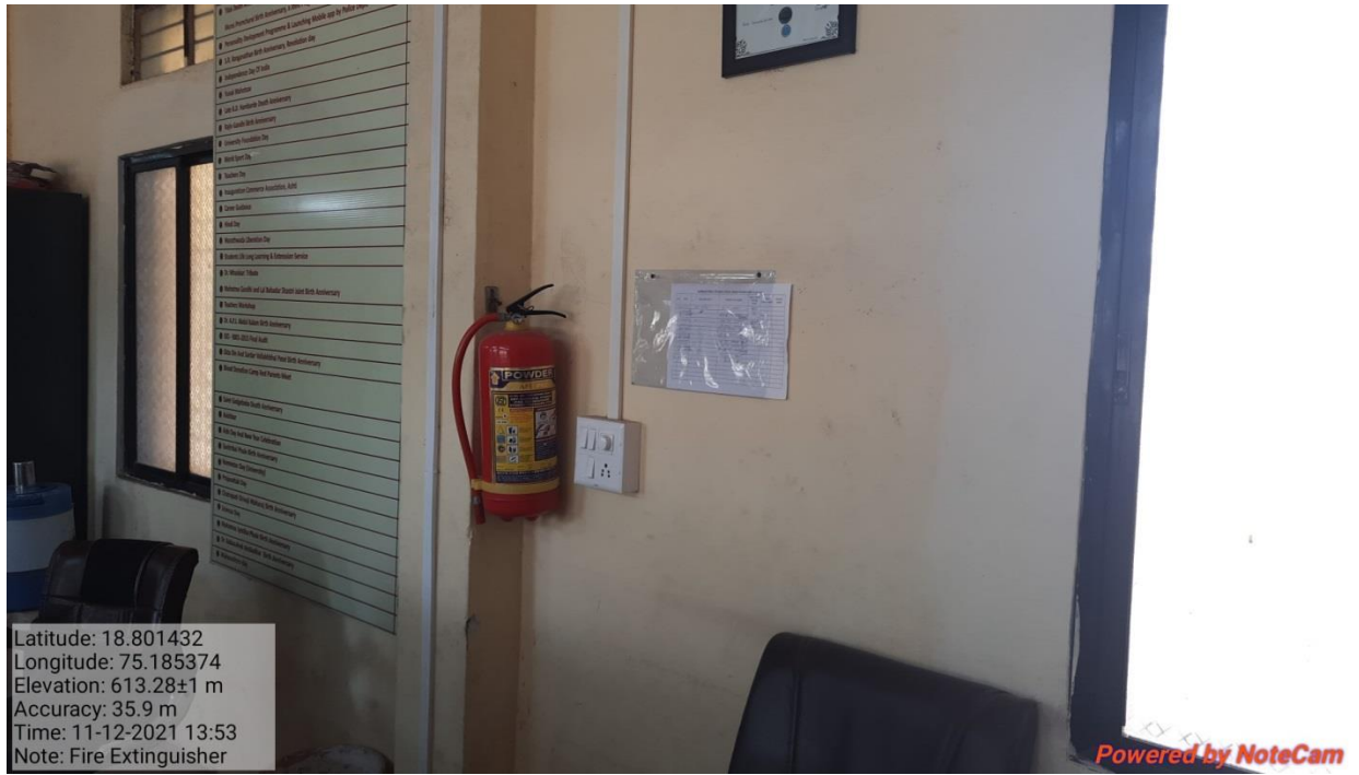
Office Fire Extinguisher
