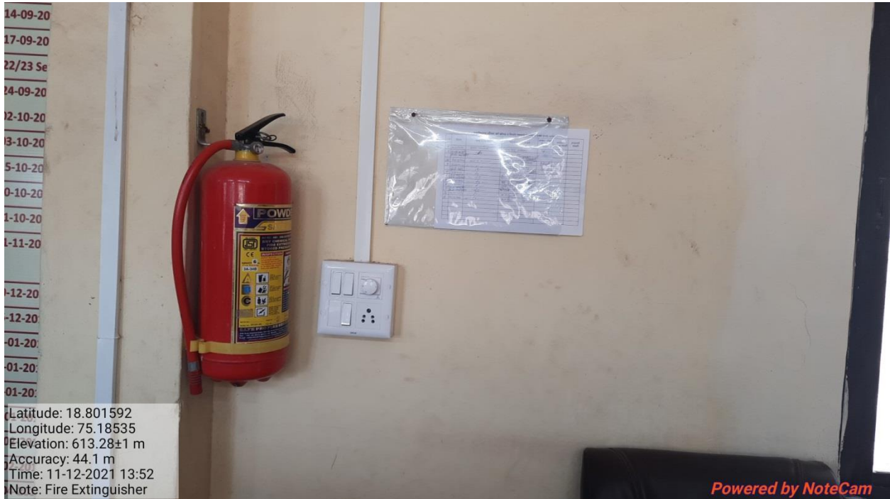
Office Fire Extinguisher
