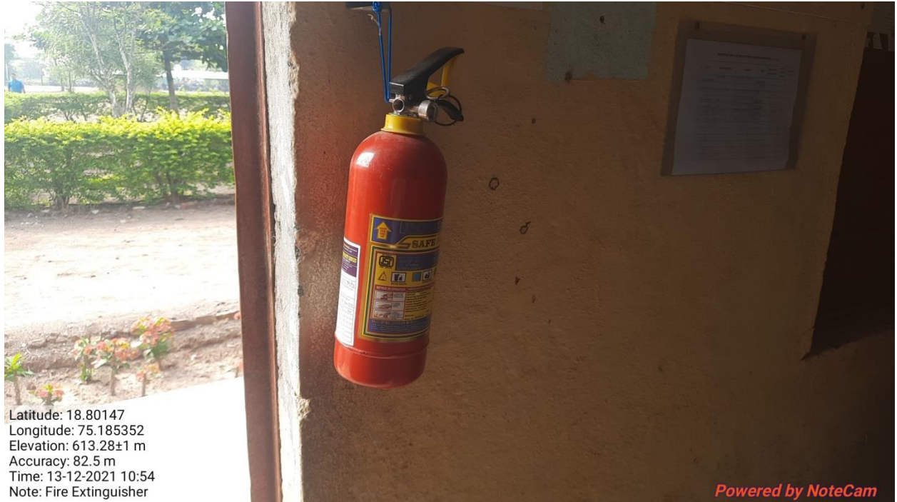
Chemistry Lab Fire Extinguisher
